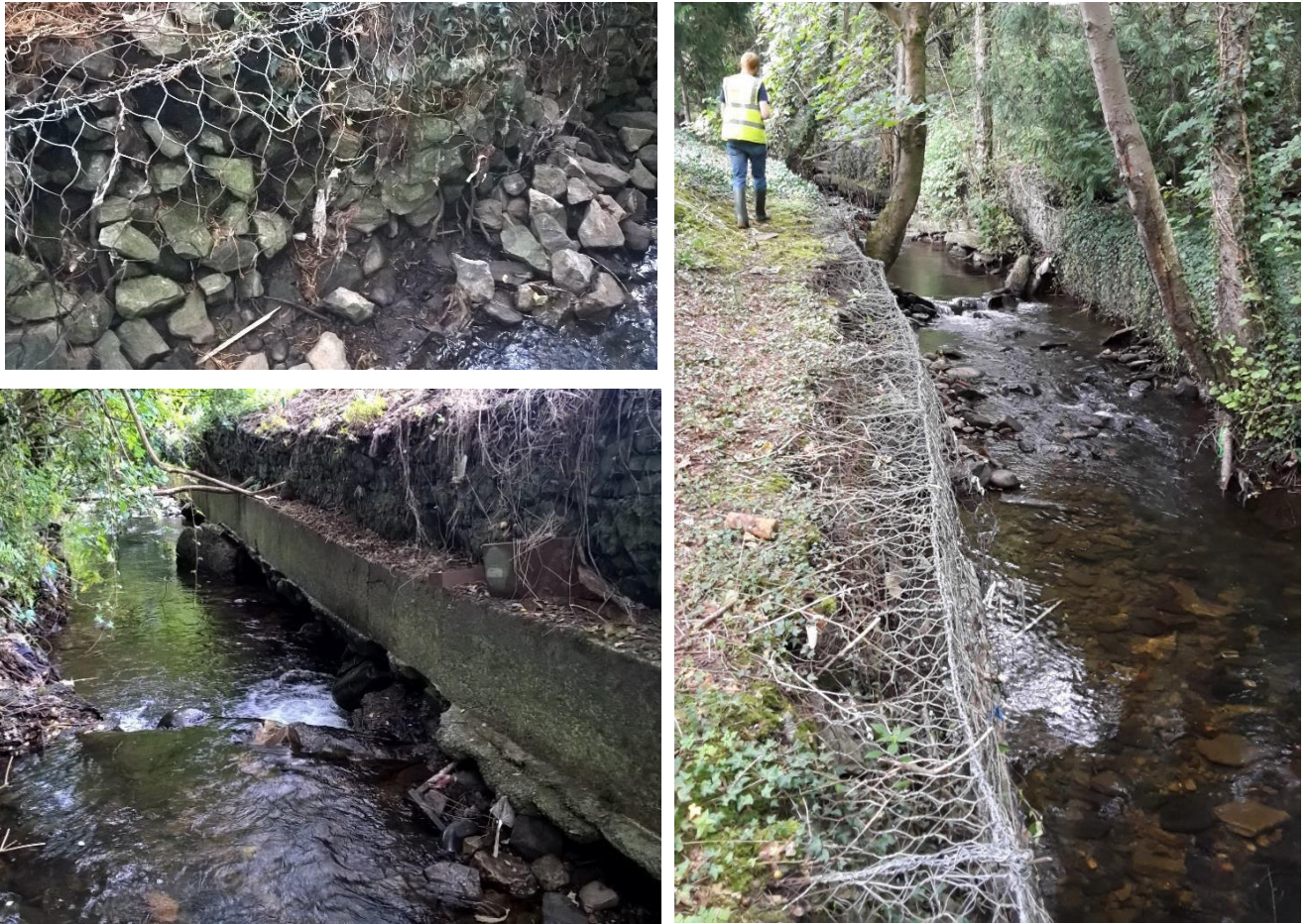
Figure 5 – Section 3: Typical photos of banks affected by scour
