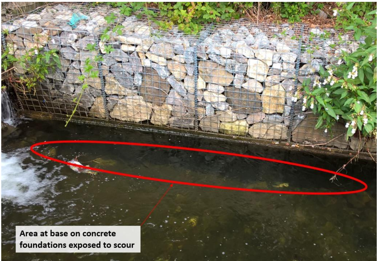
Figure 4 – Section 2: Gabion foundations exposed to scour
